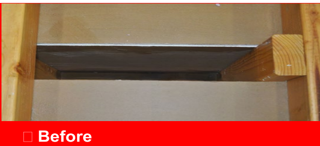
Wall cavities are open to attic
