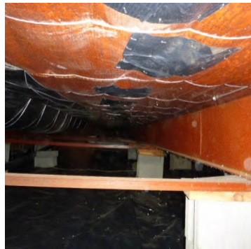
Blow holes in belly material patched.
