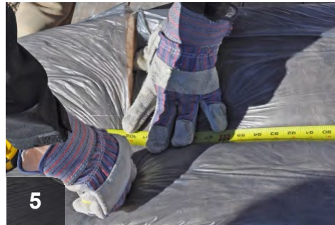
5 Measure batt to length of cavity with extra for overlap from stuffing tool
