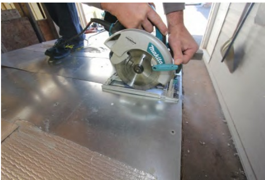
Another option: cut the roof open along the highest point from end to end. Make crosswise cuts at each end if needed
