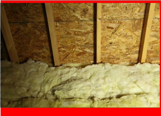
Insulation should not block vented eaves
