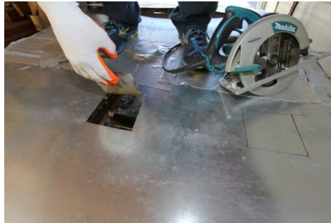
Cut a hole into each truss cavity, big enough to inspect the opening and admit the fill tube
