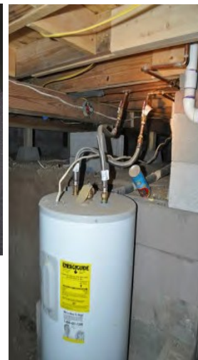
Adjust water heater settings and insulate as needed
