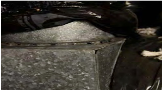
Seams, cracks, joints, holes and penetrations that are 1/4-inch or less
