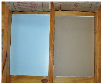
Option 1, Cover openings with rigid material, either XPS or drywall
