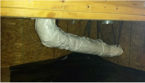
Supported and Insulated dryer vent through unconditioned space. Venting slopes downward toward termination.
