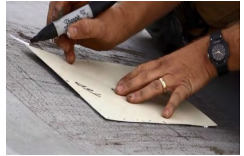
Use a 10"x10" sheet metal patch to mark the center of the hole.
