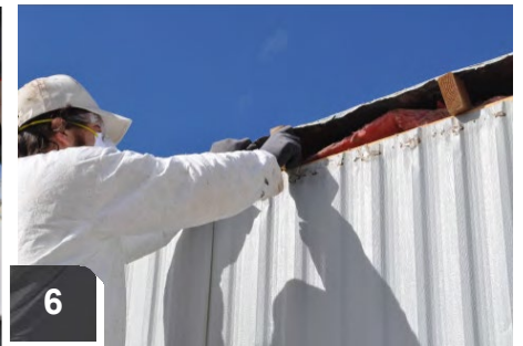
Place blocks to lift roof and enable inspection of roof cavity for obstructions and other concerns
