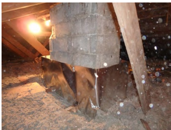
Damming is held in place with mechanical fasteners and maintains 3" clearance from chimney.
