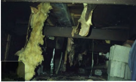
Belly damage: rodent barrier and insulation are damaged, revealing a main supply duct known as a trunk.
