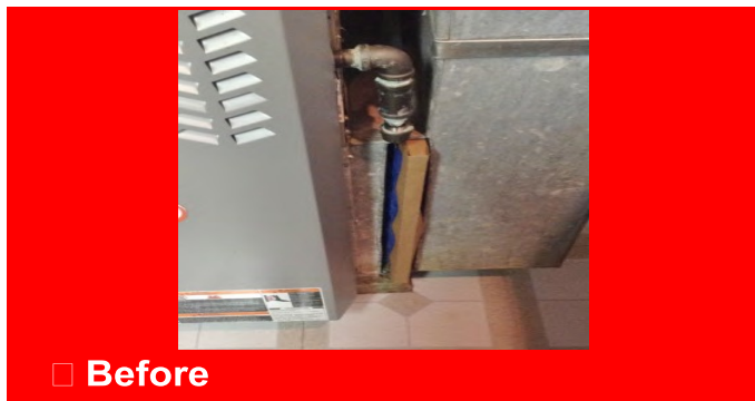
Uncovered filter slots are a point of leakage
