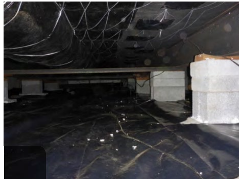
Pin up sagging belly material to prevent installing excessive amounts of insulation material.
