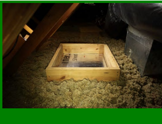
Hatch cover or panel access door should match r-value of attic insulation
