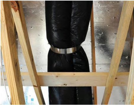
BAD: Make sure supports DO NOT compress insulation or duct
