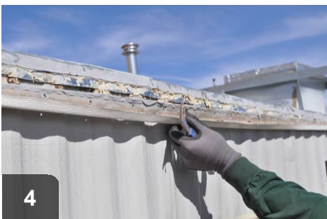
Work in manageable sections to minimize roof damage. One section of J-channel is a long enough area
