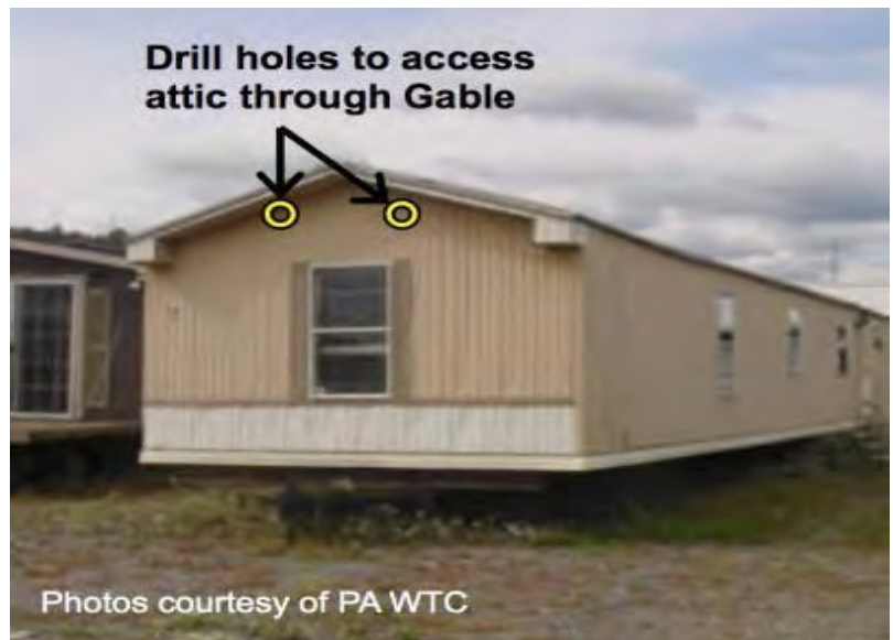
Locate the ceiling level and truss framing prior to drilling through gable siding.
