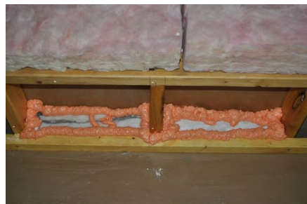
Option 4: Bridge cavities at new ceiling level with wrapped batts and SPF
