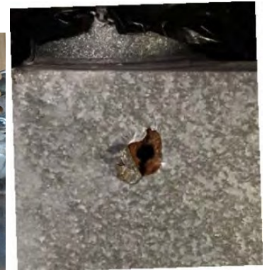
Large hole greater than 3/4" in duct or .
