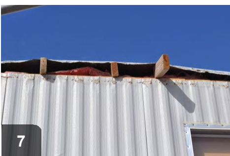
Work in small sections to minimize flexing of roof and risk of wind damage
