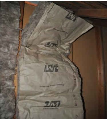
Where existing insulation is improperly installed, fix it
