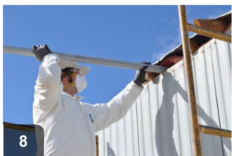
Once visual inspection has shown roof cavity to be viable, begin blowing insulation
