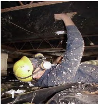
Holes are cut through rodent barrier (belly material) to insert insulation blow hose.
