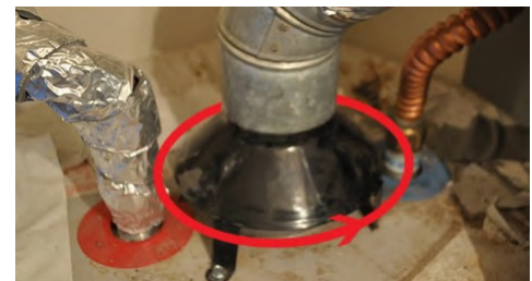
Test for spillage on all sides of draft diverter
