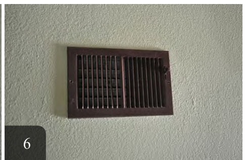
6 Once mastic is set, grill can be replaced and mastic should not show
