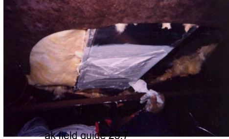
Mobile home duct systems (plenum, trunk terminations) should be sealed from below prior to patching the belly.
