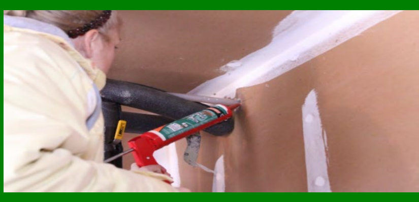
Seal penetrations to minimize risks and air leakage from garage to house
