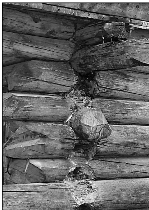
Damage from rot
