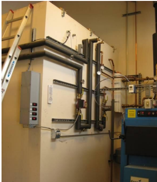
Figure 4: CCHRC's wood-fired boiler sits next to a 1500 gallon storage tank of water.
