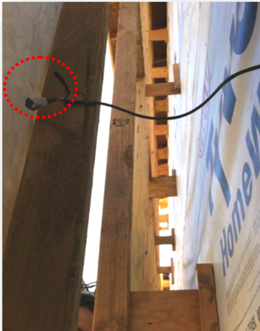
Figure 7. Temperature (black) and humidity (white) sensors were installed on the interior side of outer membrane.
