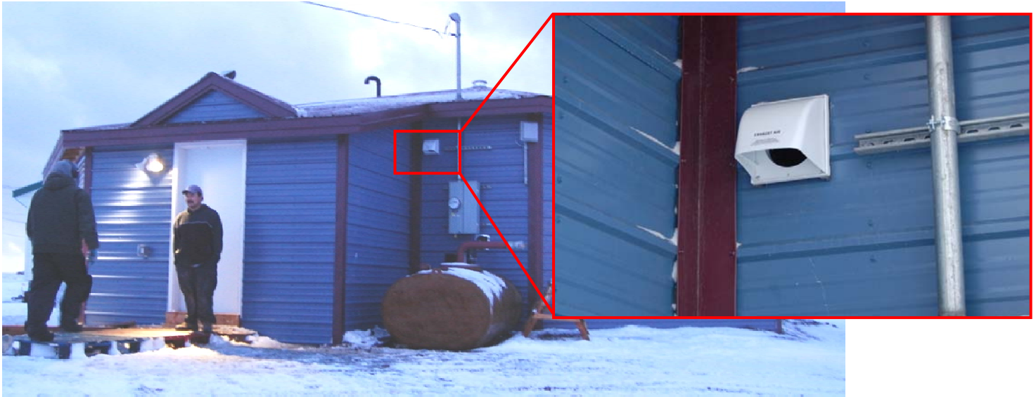
Figure 16. Outside corner near the floor moisture sensor. The sensor is at the bottom of this wall where the Arctic entry joins the main house of the wall. There are several plumbing and electrical penetrations in this portion of the wall. The inset is a close up of snow driven into the corner after a storm in December 2010.
