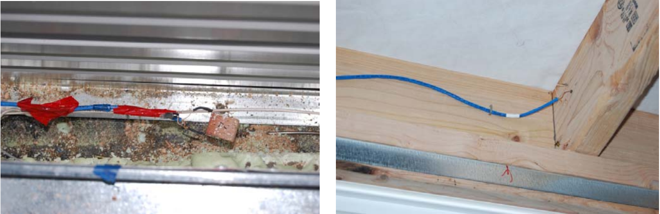
Figure 12. Installation of moisture sensors in Quinhagak. The roof used wooden trusses, but the walls were all metal and spray foam. Notice the wooden pins are not in line with the grain of the wood, an installation error that could affect the calibration of the sensor slightly.
