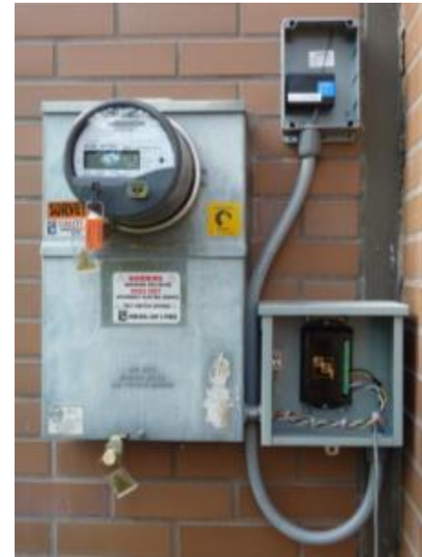
Electric Meter (Chugach Manor)
