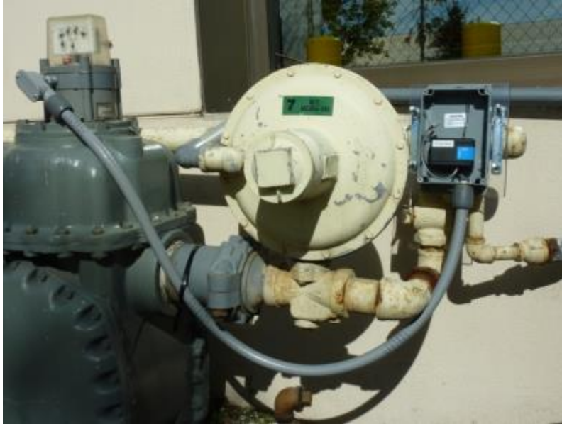
Gas Meter (AHFC Headquarters)
