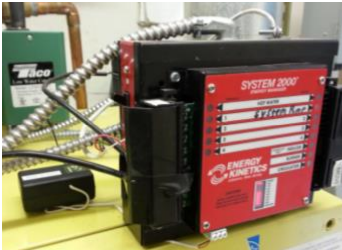
Boiler Alarm (Glacierview, Seward)
