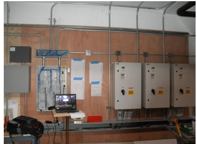
DDC boiler controls and VFD Pump Controls
