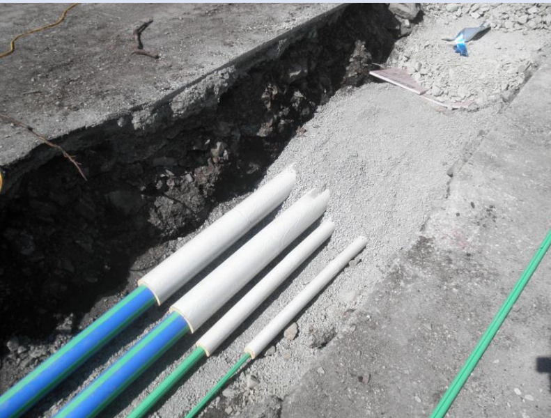
Hydronic distribution and domestic hot water distribution piping
