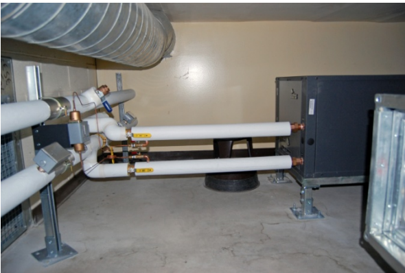
Supply and return pipes connect a heat pump to the ground loop.
