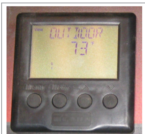
A modulating aquastat will change the output temperature of a boiler based on the outdoor temperature.
