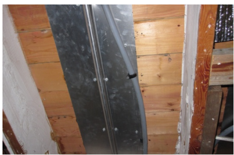
This "staple up" radiant floor system uses metal connectors to help distribute heat to the floor. View from basement.
