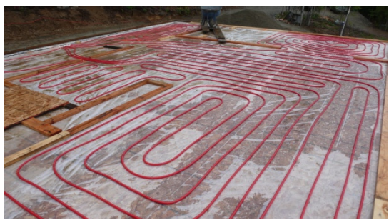
PEX tubing is laid out for radiant flooring before concrete is poured.
