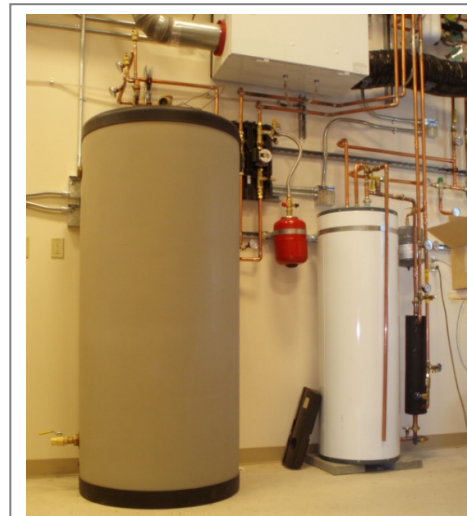
A 120-gallon tank and a 50-gallon storage tank hold water.
