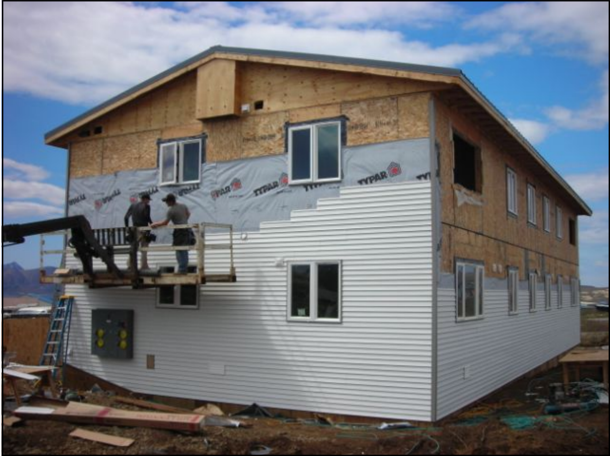
Siding is applied to a teacher housing 4-plex in Sand Point, Alaska in 2007.
