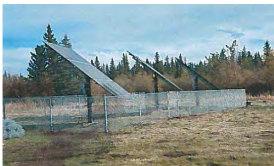
Solar arrays at Tazlina Apartments that will service three duplexes.
